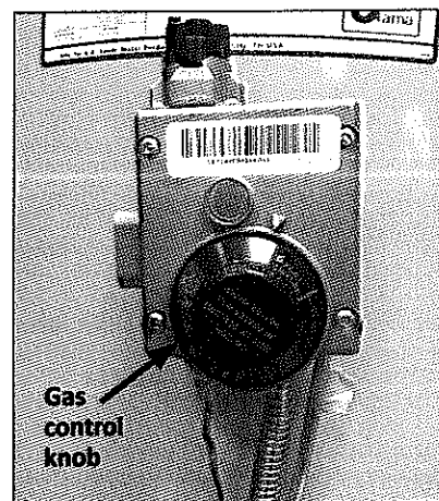
Figure 17 - Turn gas control/temperature knob OFF.
