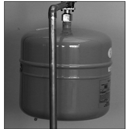
Figure 12 - A Thermal Expansion Tank helps protect the home's plumbing system from pressure spikes.
