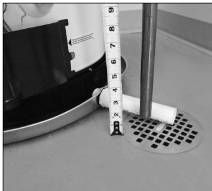
Figure 26 - Temperature and Pressure Relief Valve Pipe
