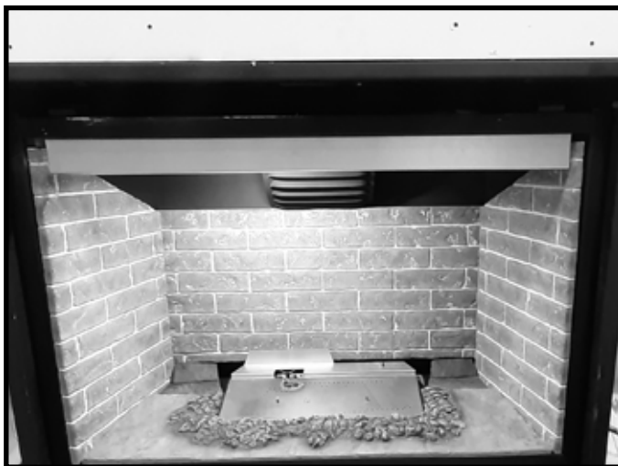
Figure 9 Refractory Kit Installed
