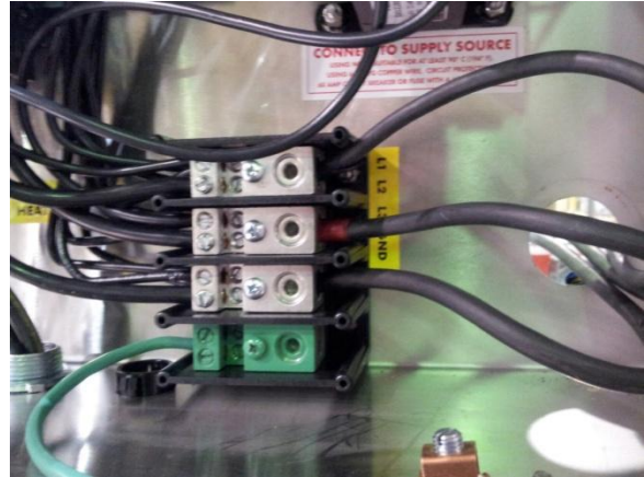
Main distribution block for 44's incoming 3-phase
