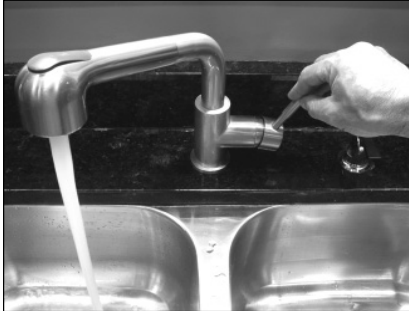
Figure 40 - Let the hot water run until it is cool.
