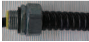
Figure 99: Example of Conduit.
