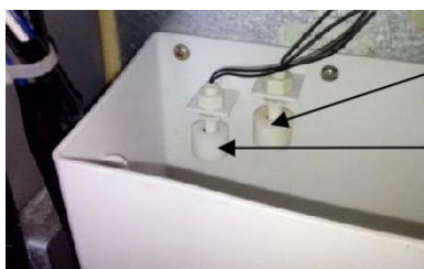
Water level switch 2 Water level switch 1
