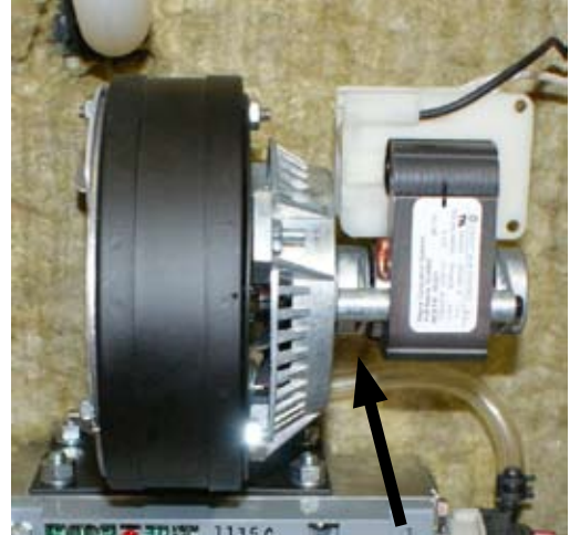
Fan Pressure Switch Hose
