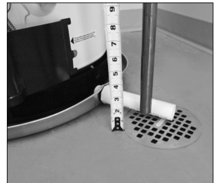
Figure 26 - Temperature and Pressure Relief Valve Pipe
