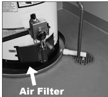
Figure 24 - Filter attached to water heater.
