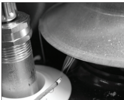
Figure 32: Test the air supply and vent to make sure the water heater has adequate air and is venting properly.
