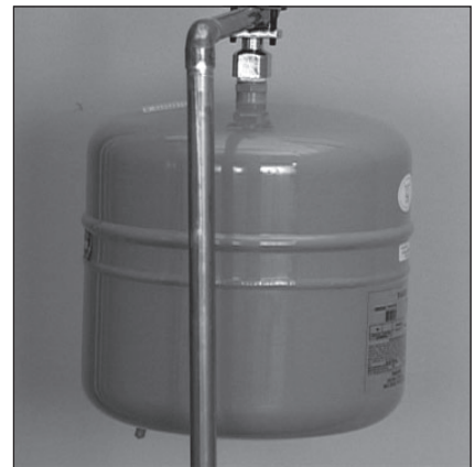
Figure 22: The Thermal Expansion Tank should be pressurized with air, using a hand pump, to match the home's incoming water pressure.
