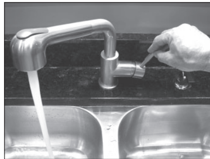
Figure 10: Let the hot water run until it is cool.
