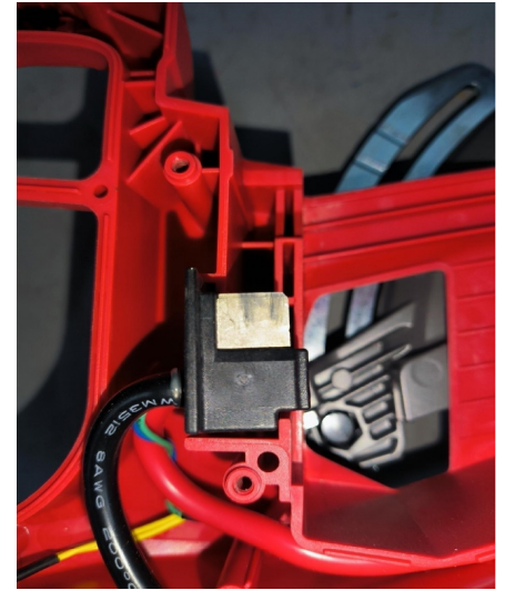
6) Closeup of Battery Terminal Block and wires.
