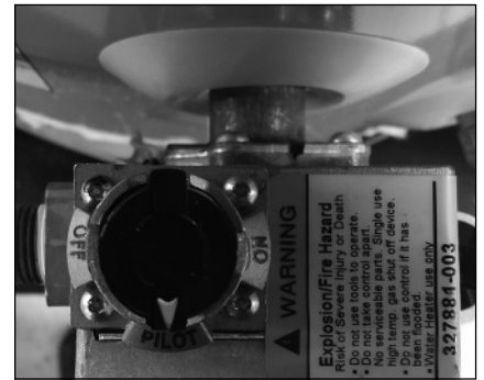
Figure 34 - Gas control/valve top view.
